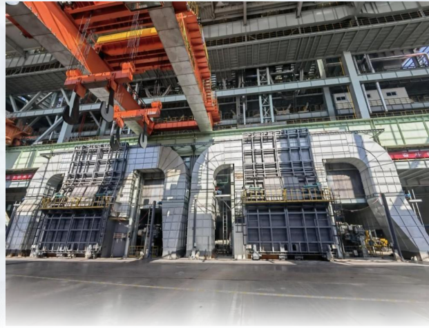
Shangang Group Energy Power 110kV Transformation Project
